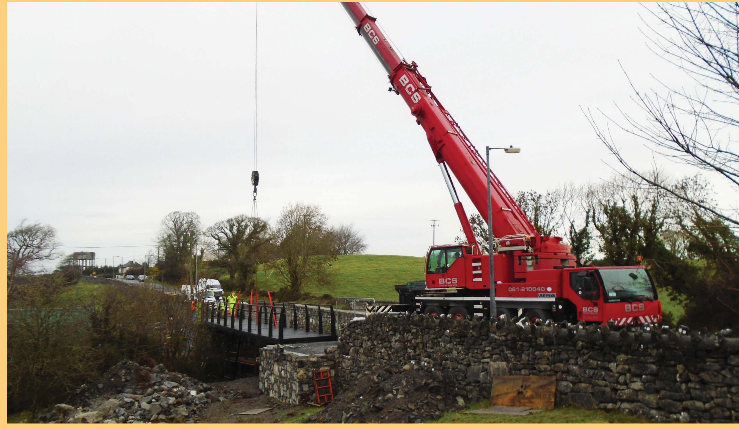
Installation of footbridge at Tuam Road, Headford, 2018 (Galway County Council) Suiteáil droichid choise ag Bóthar Thuama, Ath Cinn, 2018 (Comhairle Chontae na Gaillimhe)
